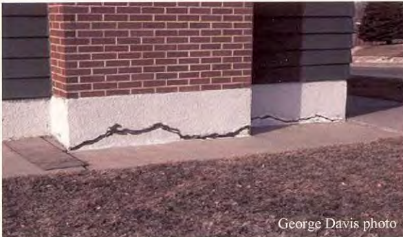
Cracked foundation caused by heaving clay soil
